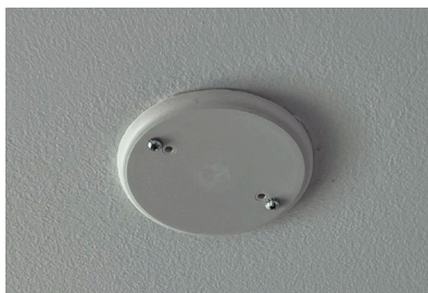
Wire & Brace For Future Ceiling Fan
